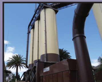
Conveyor Transfer Points
