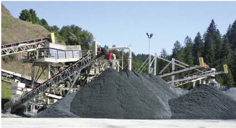
Above: Mark West Quarry Wash Plant. Top Right: Aerial view Santa Rosa Plant. Right: Diemme filter press.
